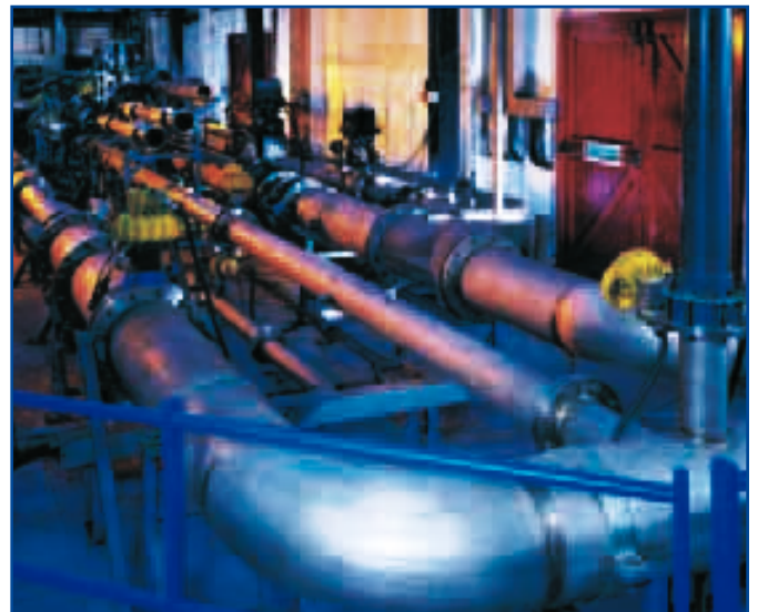
Flowmeter calibration rig
