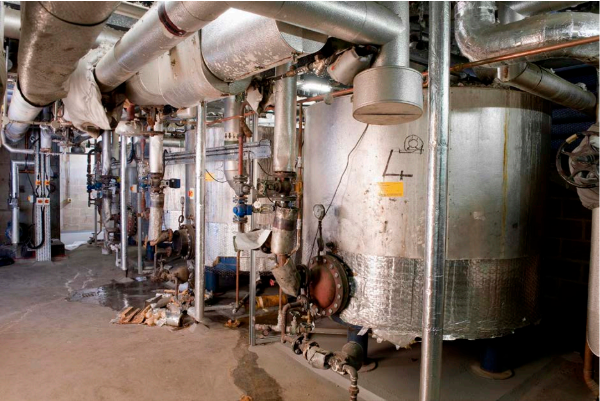
St George's Hospital plant room before the upgrade
