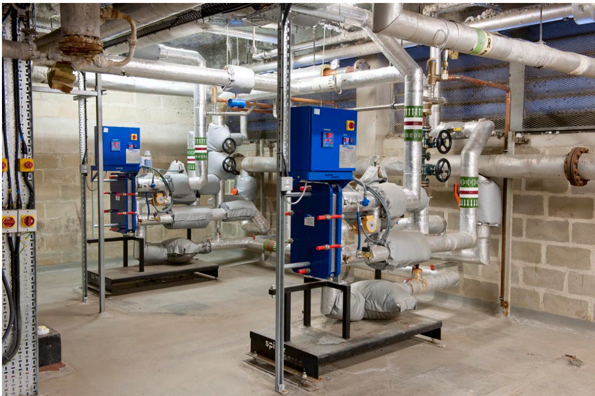
St George's Hospital upgraded its calorifiers to Spirax EasiHeat plate heat exchangers
